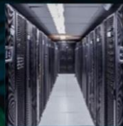
Delta HQ IT Data Center LEED V4 ID+C Platinum
